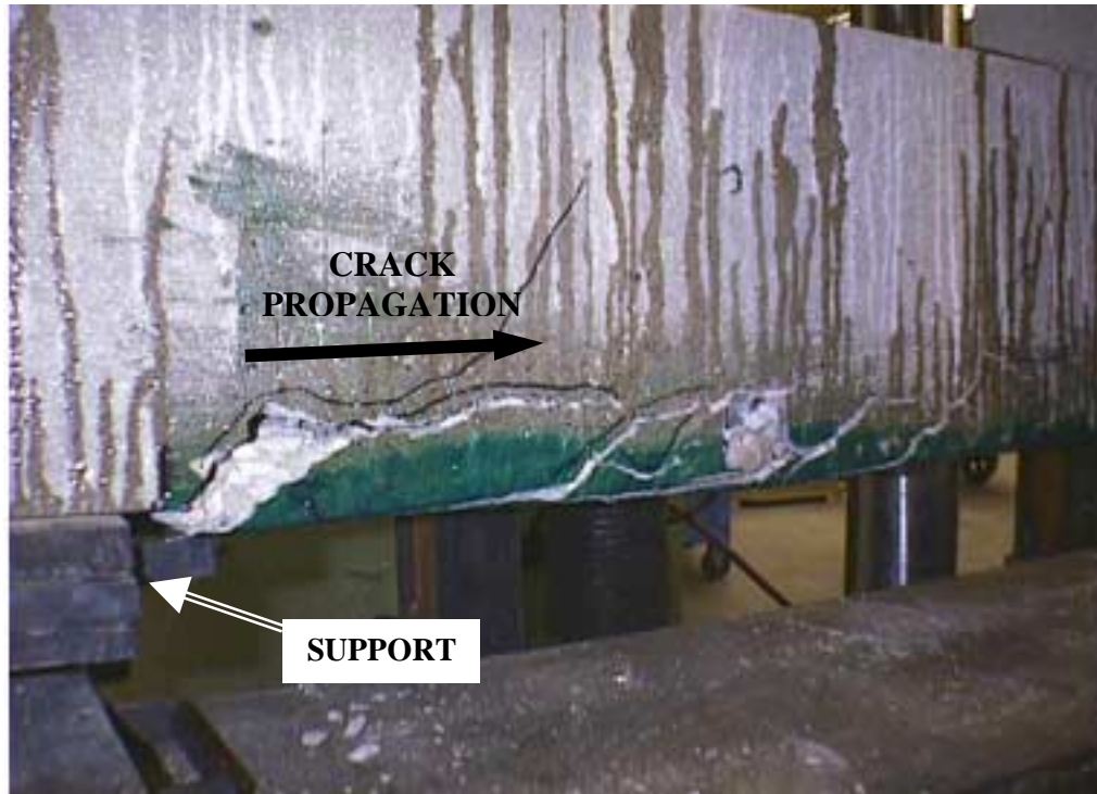
Figure 1. Concrete Cover Delamination – Failure Mode I (Beam A3)
