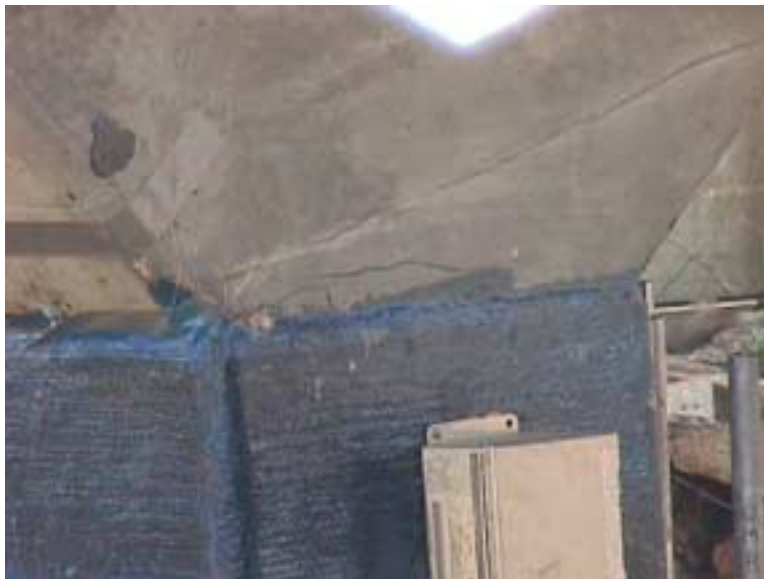
(b) Cracking at the top of the column.
