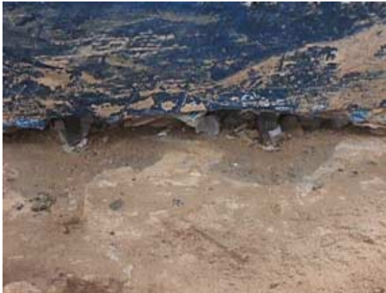
(a) Rupture of FRP rods at the base of the column.
